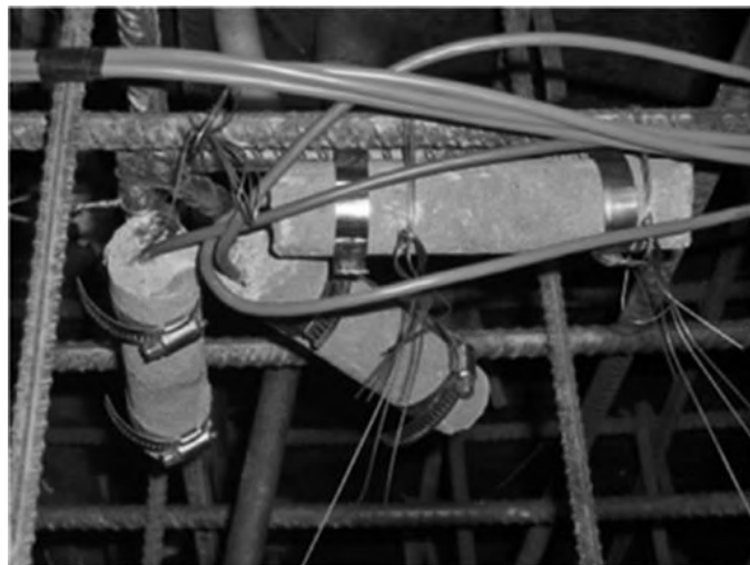
Figure 4: Vibrating wire strain gauges (Geokon Model GK4200) installed at the inner tube of Canton Tower.
